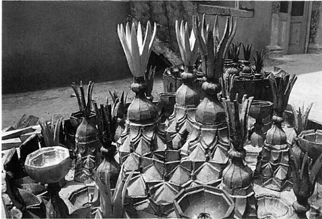
The Ochrida synagogue: The central decorative part of the wooden dome during renovation.
